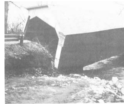
The flood of 1977 almost destroyed the Eagleville Bridge. Quick action by County DPW diverted the river and saved the bridge. The flood waters ero the east abutment. The west abutment rests on bedrock and was unaffec Photos courtesy of the Washington County DPW.
